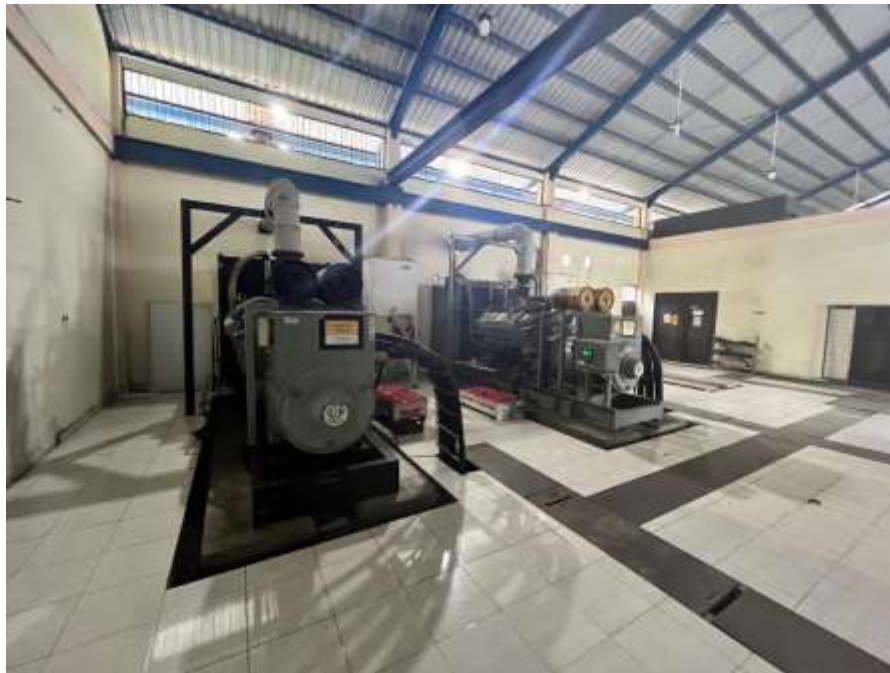
Figure 1. The standby generator units installed at sentani international airport.
